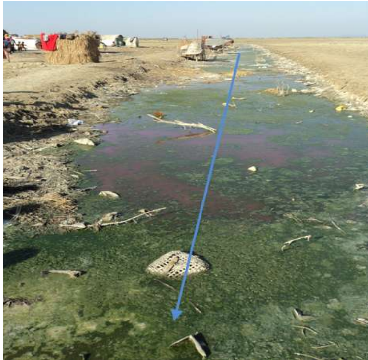
Fig. 16: Silted tidal channel to be rehabilitated
