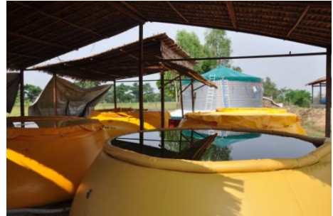
Figure 5: Oxfam 30m 3 onion tank for water treatment.
