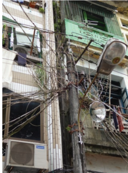
Figure 19: Distribution system in downtown Yangon 105
