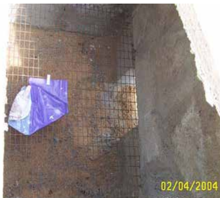
Fire grill inside incinerator
