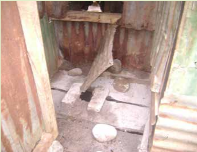
Poor quality latrine with rusty corrugated sheet walling, posing a health and safety hazard
