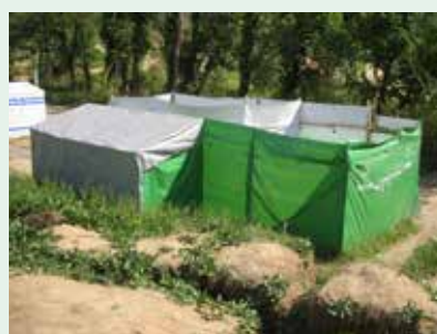
Screened latrine and bathing unit with internal menstrual slab and raised sides for additional privacy
