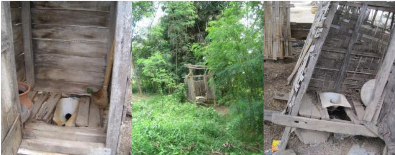
Unhygienic Latrines with Pan and Pipe
