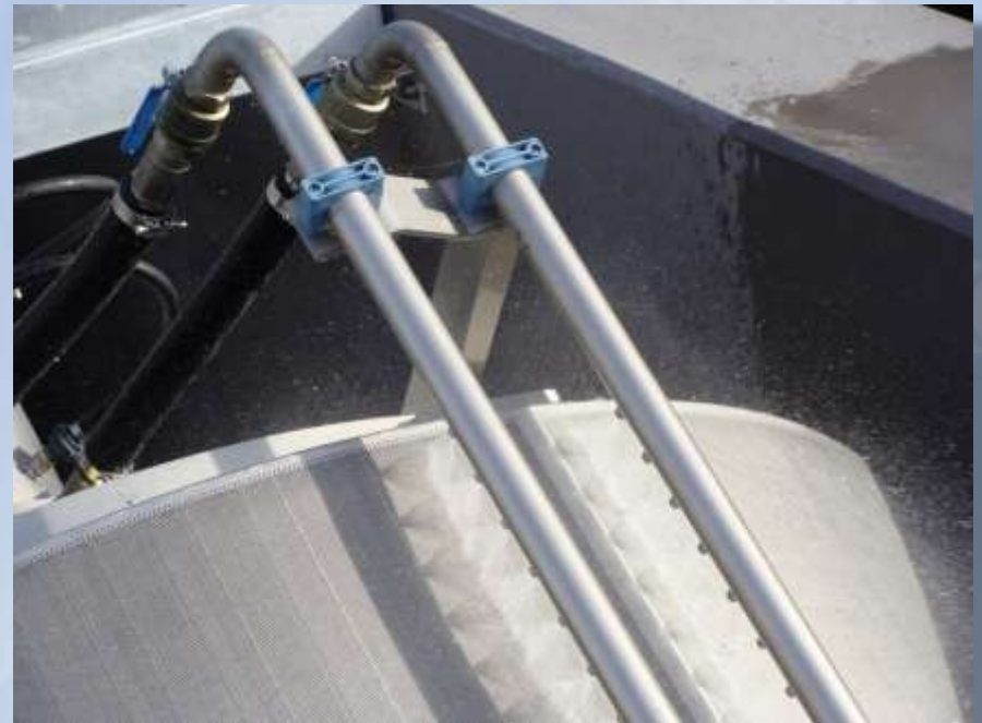
Screen drum spray bars
