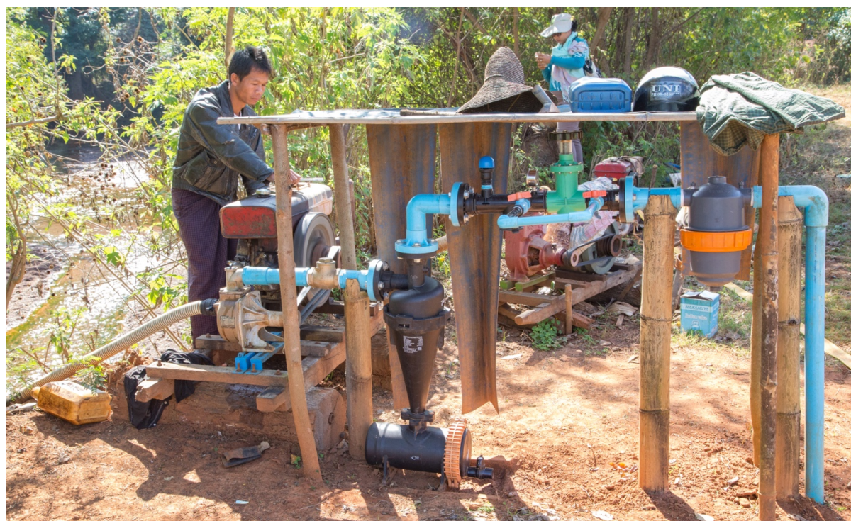
Figure 52: Prime drip system supplied water filter with hydro-cyclone, disk filter and pressure release valve.
